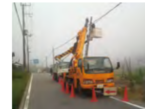
Natural disasters such as typhoons and earthquakes often cause damage to telecommunication networks. We have a system and resources in place to conduct recovery work immediately to prevent or minimize network outages.
