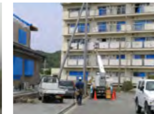
To restore networks from damage by tornadoes in May 2012, we conducted repair work for 26 utility poles and telecommunication cables at 137 locations in Tsukuba City, Ibaraki.
