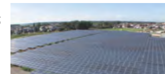
Solar power generation facilities in Sakura City, Chiba
