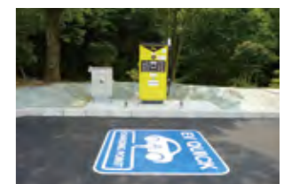
EV battery charging station on a highway
