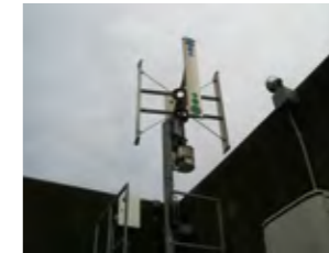
Wind power generator on the rooftop
