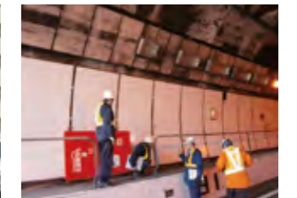
In December 2012, some ceiling panels of Chuo Express Way's Sasago Tunnel collapsed. We repaired cables of emergency telephone lines.
