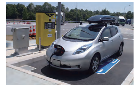
EV battery charging station
