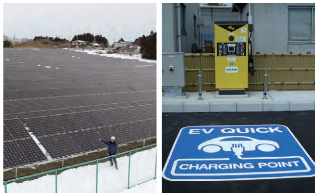
Solar power generation system
