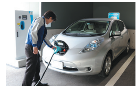
EV battery quick-charging system
