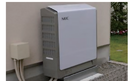
Electricity storage system for a freestanding house
