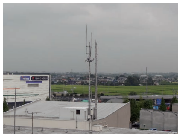
Antenna for regional government's emergency radio communications system
