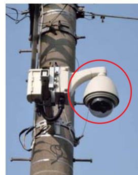
Security camera installed on a utility pole
