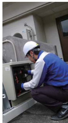
Installing smart water meters at a test station in the mountainous Hakone-machi
