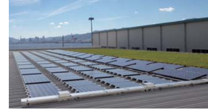
Photovoltaic Solar Power Generation Facilities of the Kobe Technical Center
