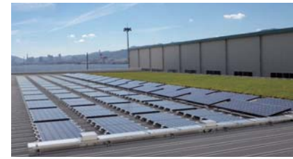
Solar Power Generator of the Kobe Technical Center
