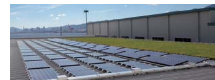
Solar Power Generator of the Kobe Technical Center
