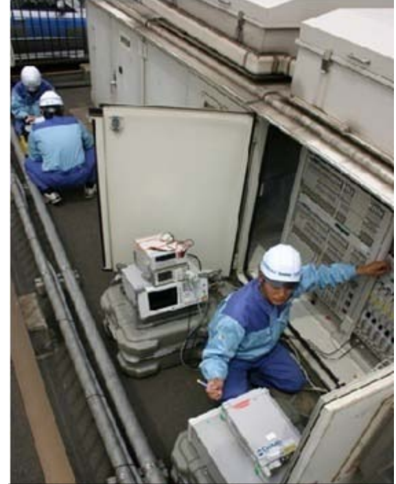
Adjustment and examination for wireless base stations (Tokyo)
