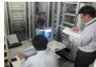
Upgrading switch programs
