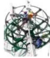
Co-installation of wireless base stations
