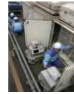
Adjustment and testing of wireless base stations
