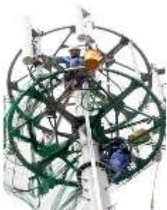
Co-installation of wireless base stations
