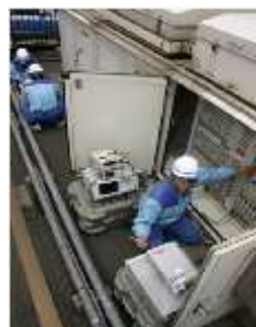
Adjustment and testing of wireless base stations
