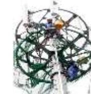
Co-installation of wireless base stations
