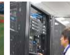
Data center maintenance
