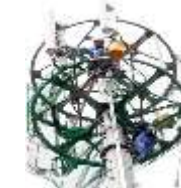
Co-installation of wireless base stations
