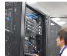
Data center maintenance
