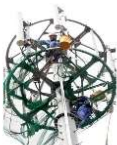
Co-installation of wireless base stations
