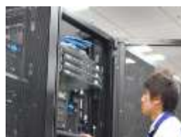
Data center maintenance
