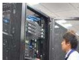
Data center maintenance
