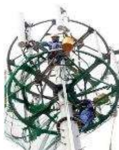
Co-installation of wireless base stations
