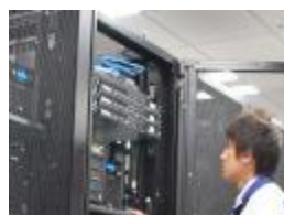
Data center maintenance
