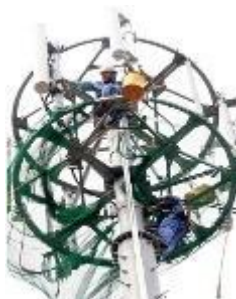
Co-installation of wireless base stations
