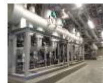
Basement air conditioning facilities
