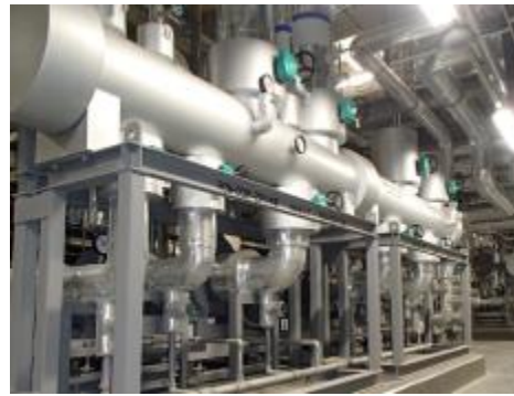
Air conditioning facilities
