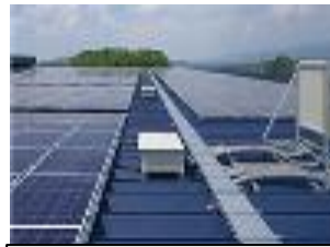
Roof-top solar panel
