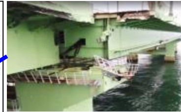
Damaged access bridge at Kansai Int'l Airport
