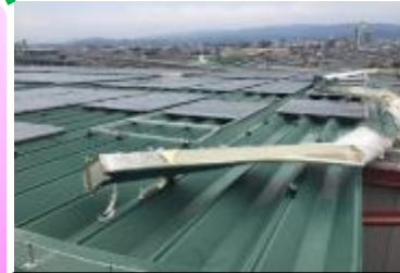
Damaged solar panels
