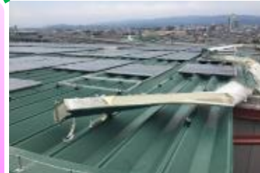
Damaged solar panels
