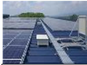
Roof-top solar panel
