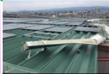
Damaged solar panels
