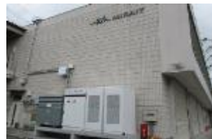
Rechargeable battery system
