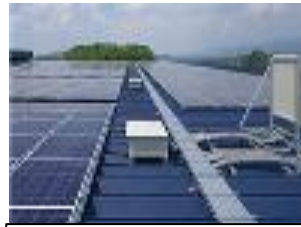
Roof-top solar panel
