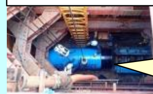
Installation of propulsion machine
