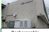
Rechargeable battery system
