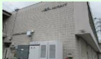
Rechargeable battery system
