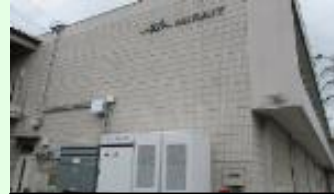
Rechargeable battery system
