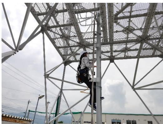
Mobile Working on a mobile antenna site
